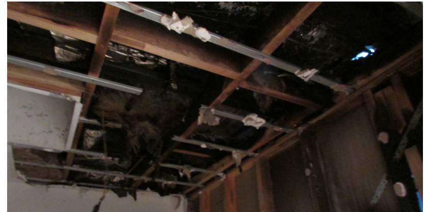
THE BLAZE DEVASTATED THE UPPER LEVELS AND ROOF AREA - AUG 30 2013
